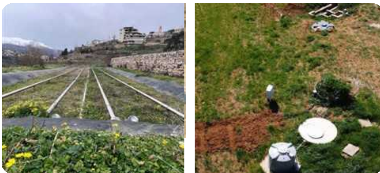
Figure 37 Decentralized Wastewater Treatment Systems (DEWATS) in Lebanon
