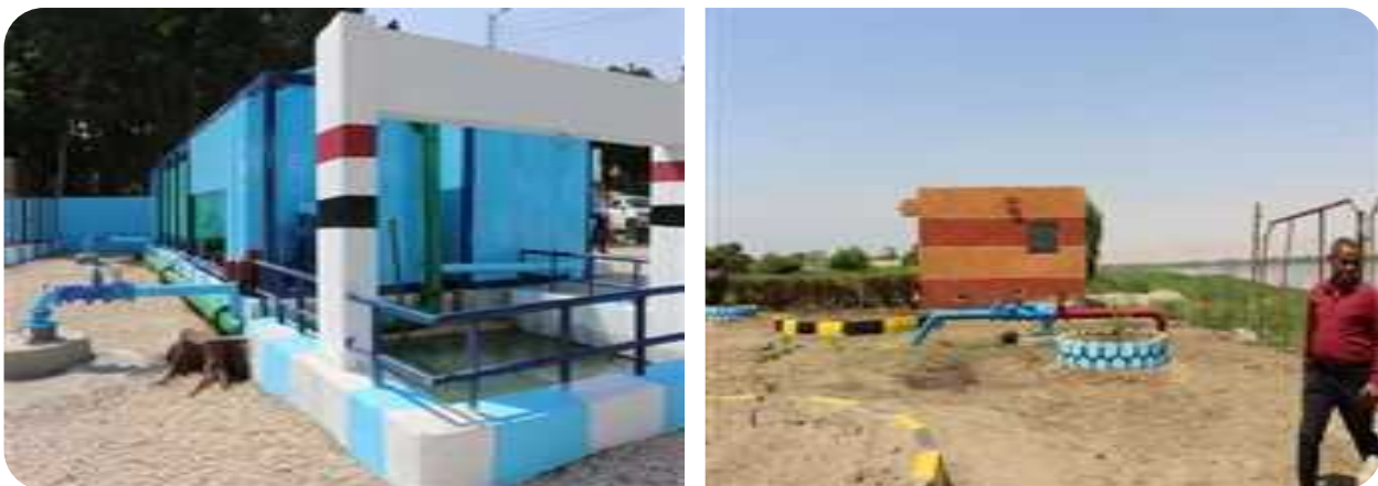
Figure 34 Pumping Wells of RBF Units in Egypt
