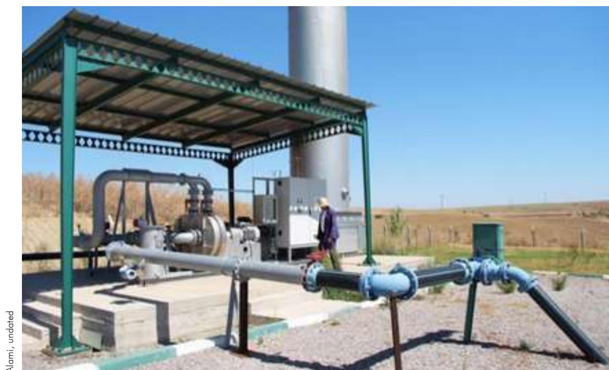
Figure 4.5: LFG collection system, Fès landfill, Morocco
