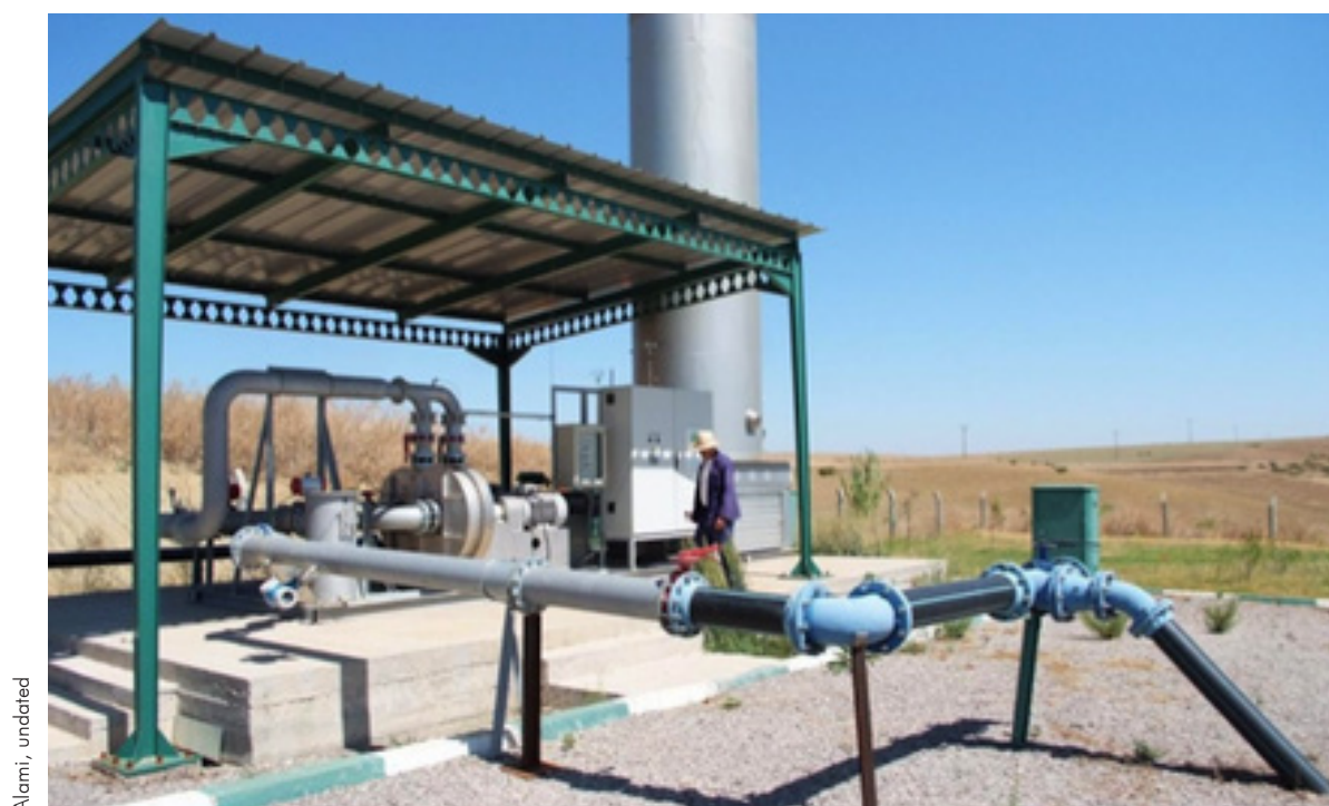
Figure 4.5: LFG collection system, Fès landfill, Morocco
