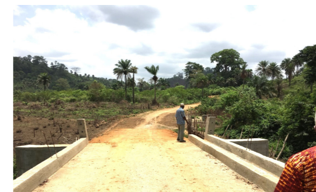
Figure-3: A crossing bridge built by the Linking Farmers to Market Project (LFM), Sierra Leone
