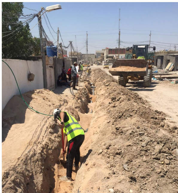
BASRA - New potable system
