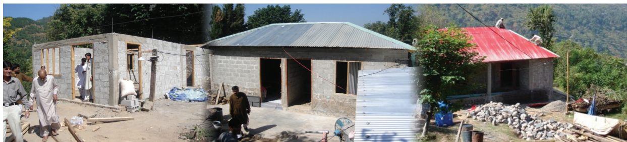
Construction of housing facilities for earthquake victims in Pakistan. The IDB has provided an assistance of $80 million.
