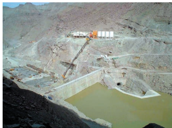
An aerial view of IDB financed under construction Jaghin Main Dam, Islamic Republic of Iran
