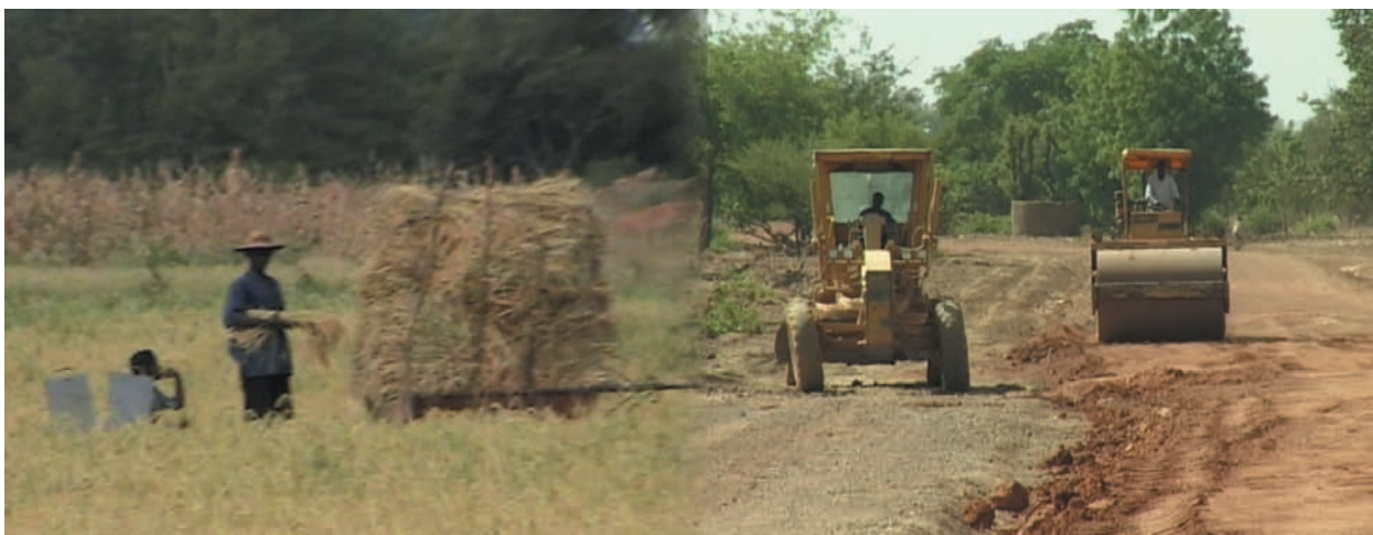
Construction of farm-to-market road network under the IDB integrated rural development project in Burkina Faso
