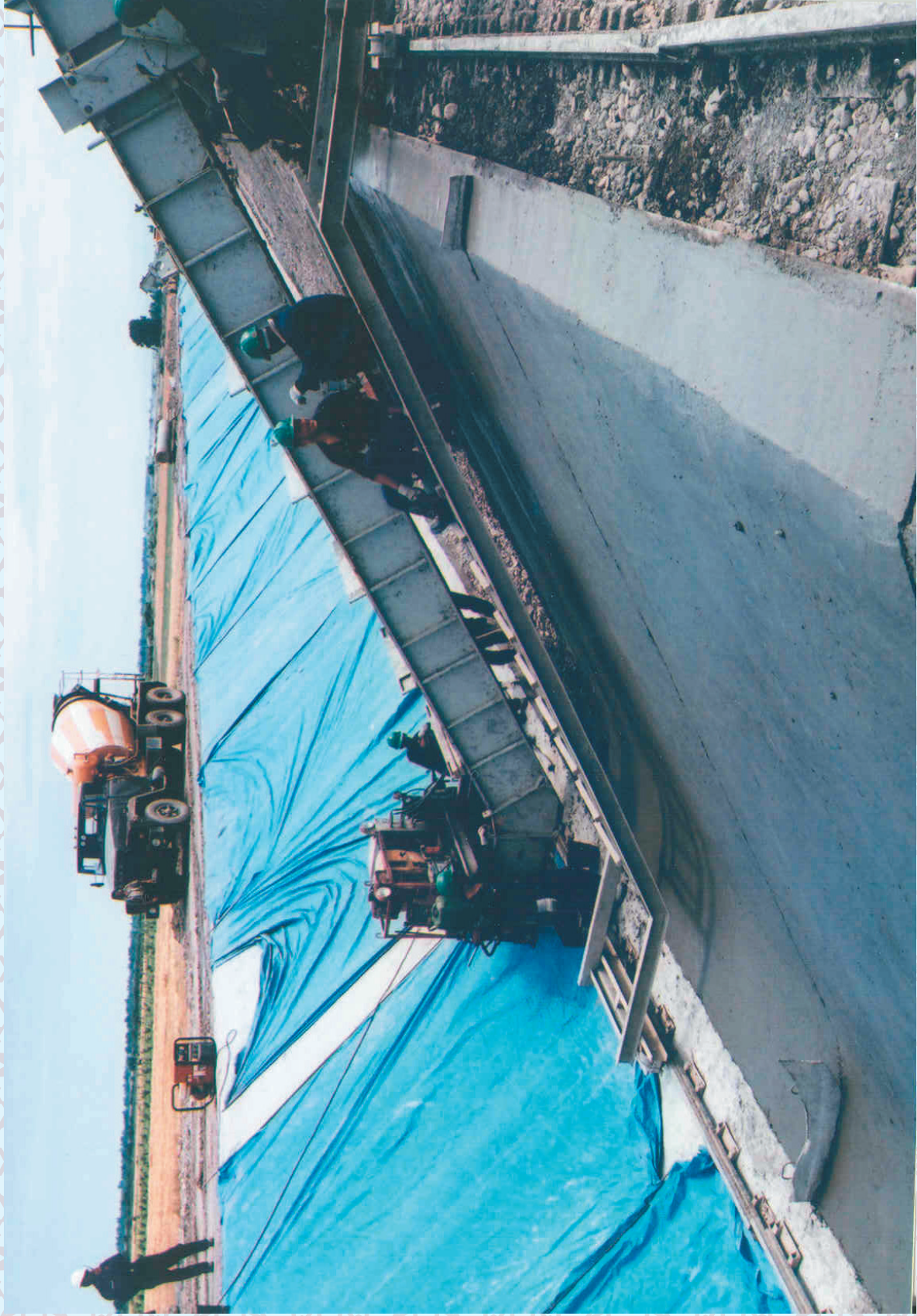
Construction of Phase-II of the IDB Financed Khanark Canal Project in Azerbaijan
